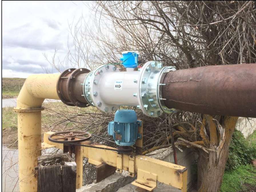
Figure 5. Picture of River Steeps Pump meter (Photo provided by OWRD).
