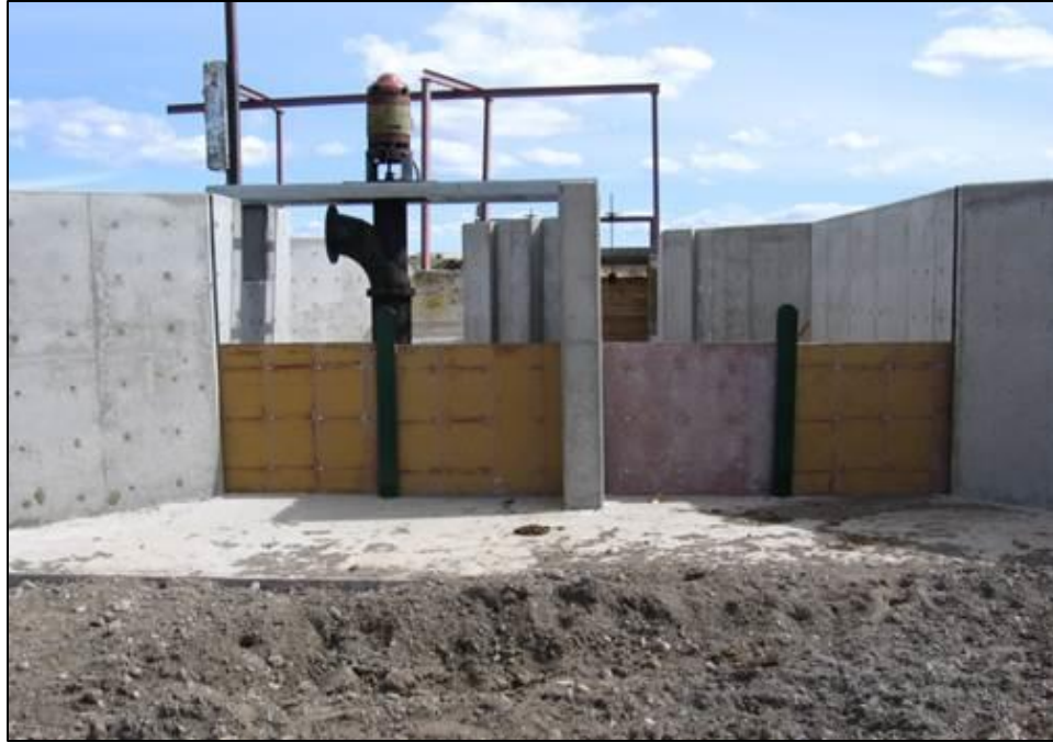
Figure 3. Picture of Crooked River Central Diversion Head Gate Structure (Photo provided by OWRD).
