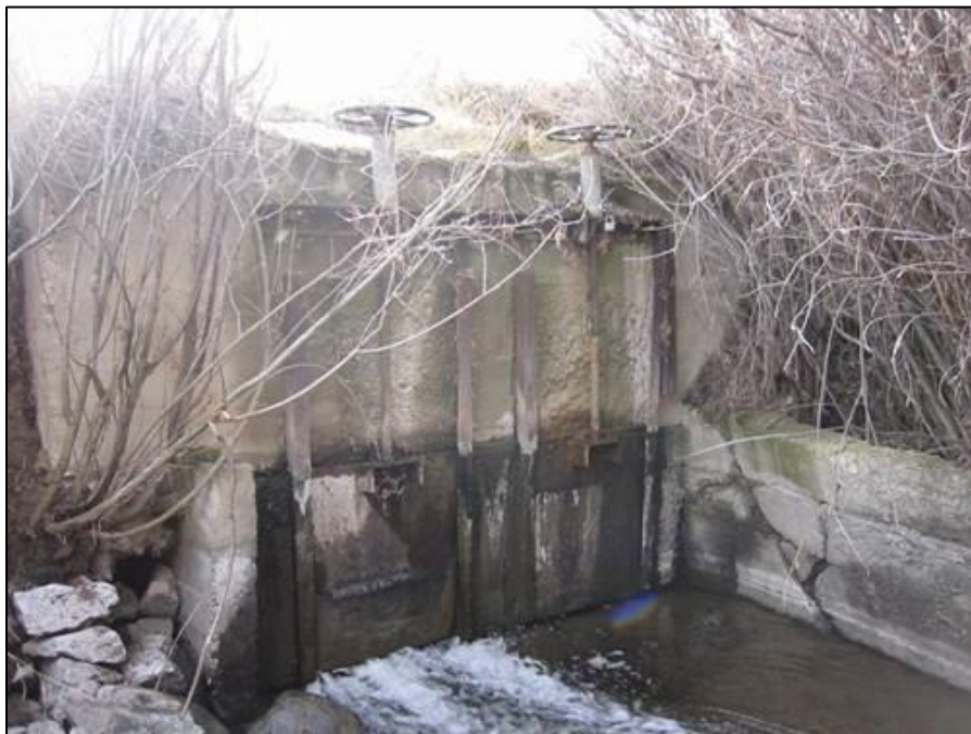
Figure 2. Picture of Rice Baldwin Diversion Canal Head Gate Structure (Photo provided by OWRD).
