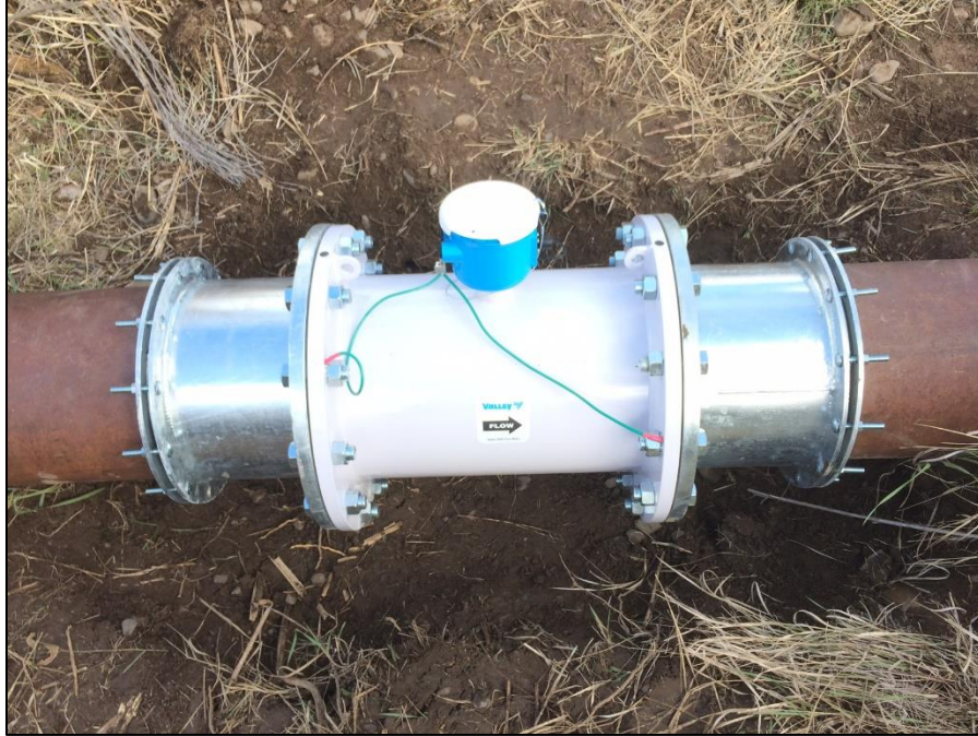
Figure 4. Picture of the Ulupalakua Pump meter (Photo provided by OWRD).
